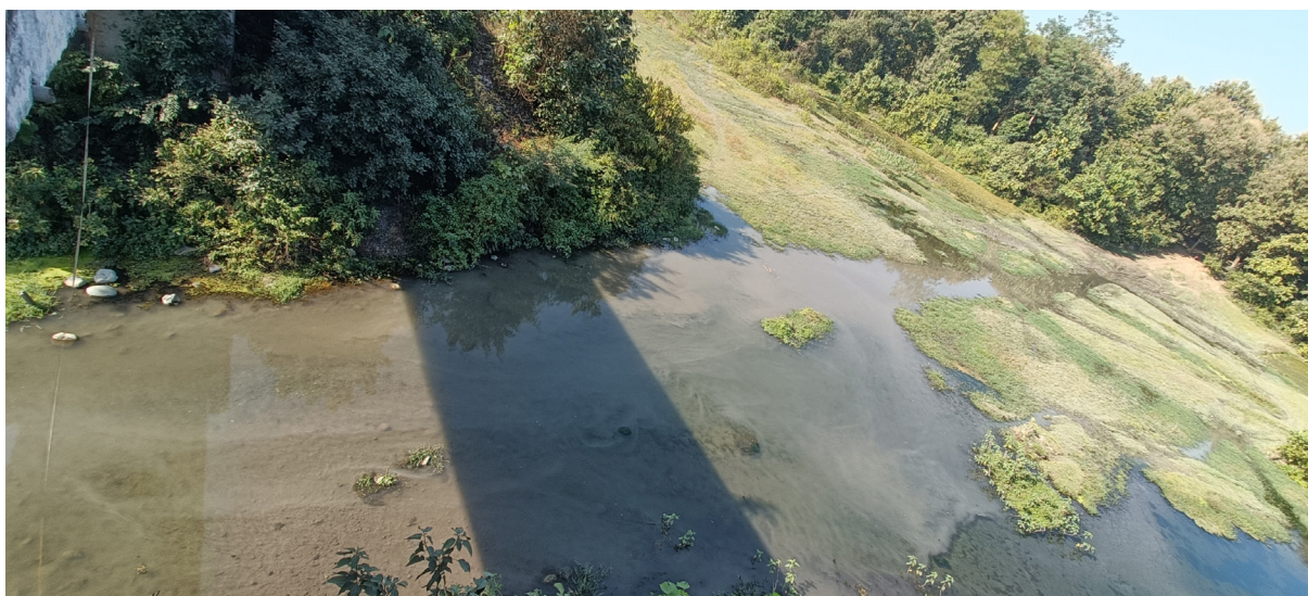
Figure 5: Water logging on both sides of the railway embankment on the Lalkuan-Chhatarpur railway track can make the drainage structures unusable by wildlife.
