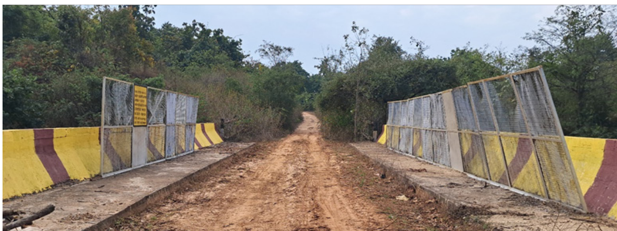
Figure 4: Existing mitigation measures need modification like barricading from the side of the overpass along the along railway track and placement of light/sound barriers
