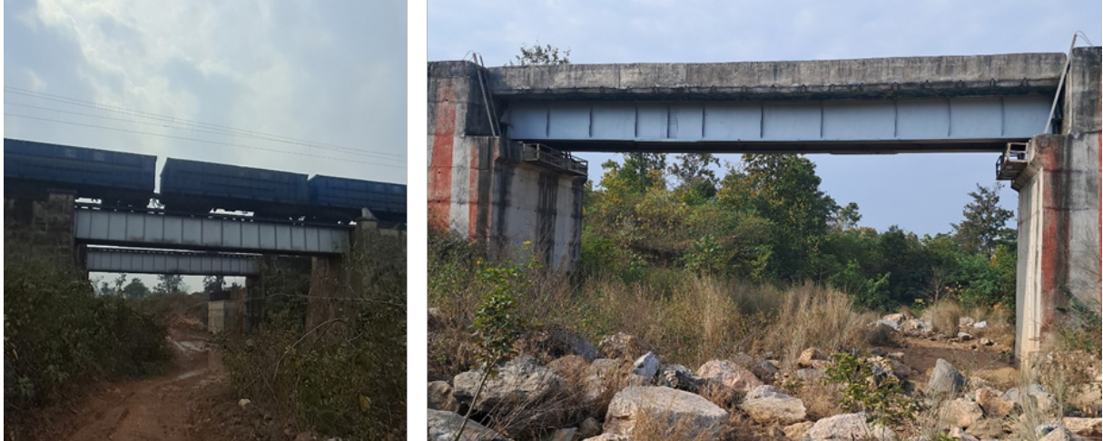
Figure 5: Existing major bridge which requires landscape modification like habitat restoration, plantation and water availability for elephant movement under bridge
