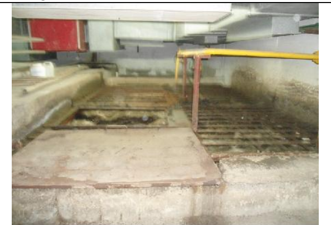
Improperly operated STP
