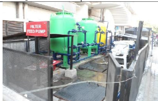
STP Installed by the Mall
