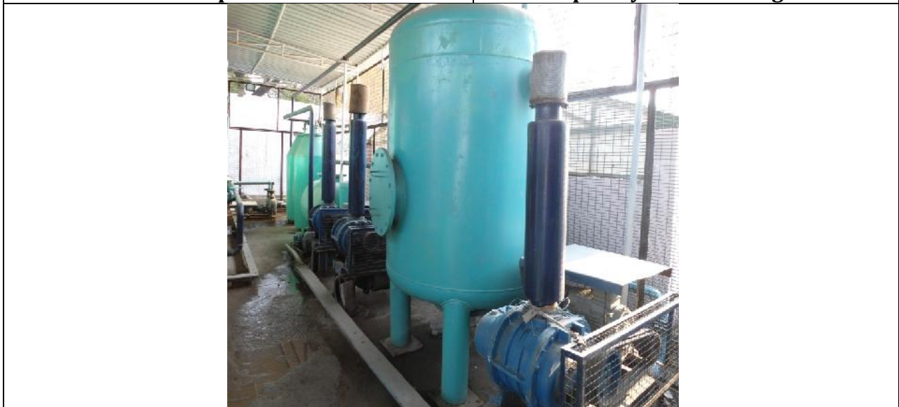
ETP installed by the Hospital
