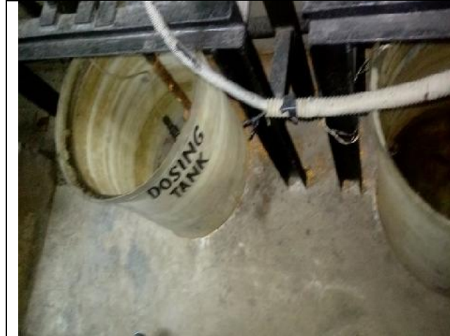
Empty chemical dosing tank of STP
