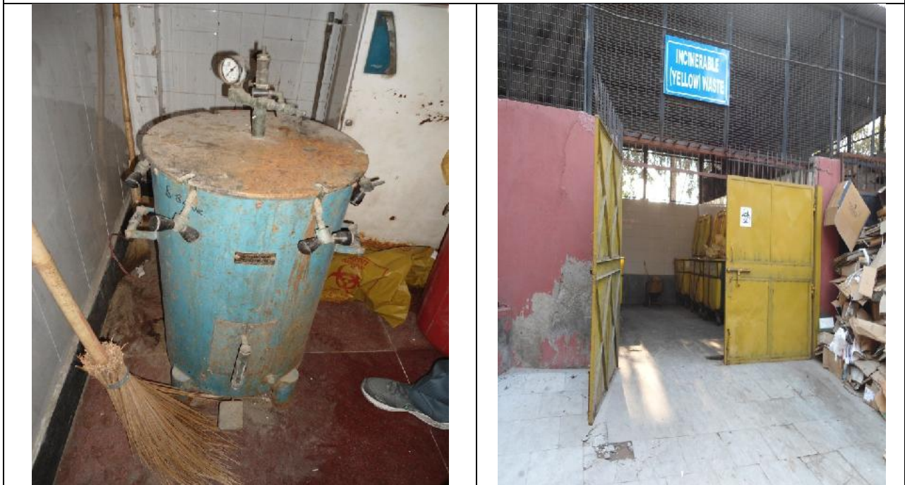
Autoclave used for pre-treatment of waste
