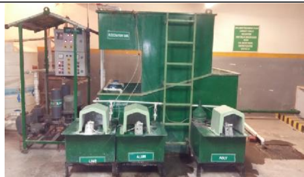
Chemical wastewater Treatment Unit
