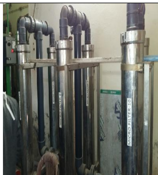
Component of STP/ETP
