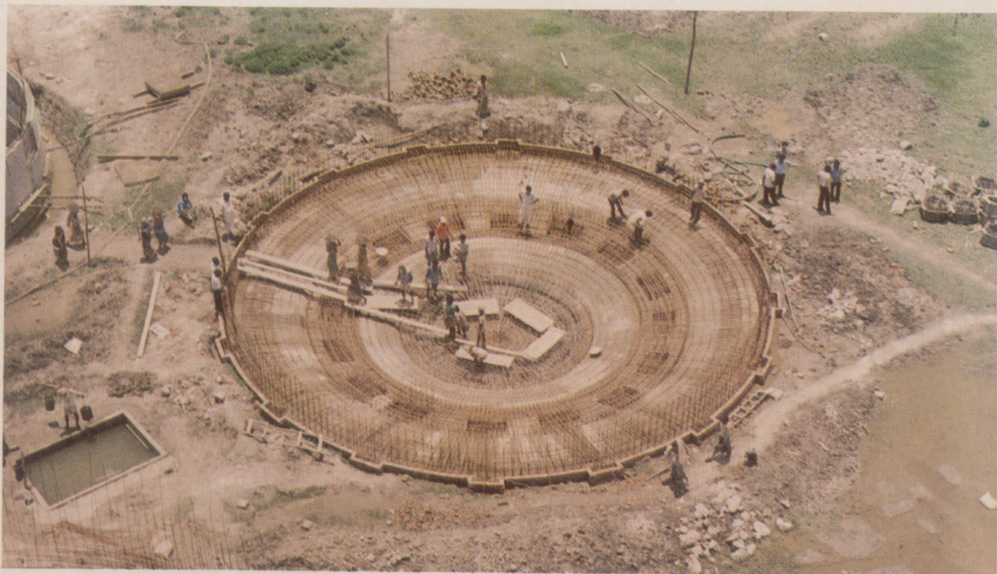
Fig 36: Construction of a Sewage Treatment Plant at Baranagar—Kamarhati under Ganga Action Plan
