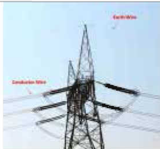
Figure 12.6. A high voltage transmission line showing the conductor wire and the partially visible earth wire that birds frequently collide with.
