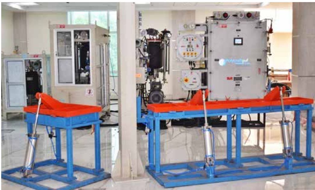
Photograph of High Pressure PU Foam Processing Unit with Moulds established at Laboratory for Advanced Research in Polymeric Materials (LARPM) CIPET, Bhubaneswar
